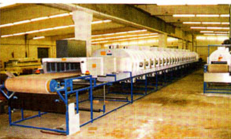
Fig. 2 MDBT 70+24 oven for microwave drying of insulation materials
